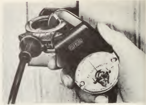
7.44. Taking the amperage reading of refrigerating unit. (Pyramid Instrument Co.)
